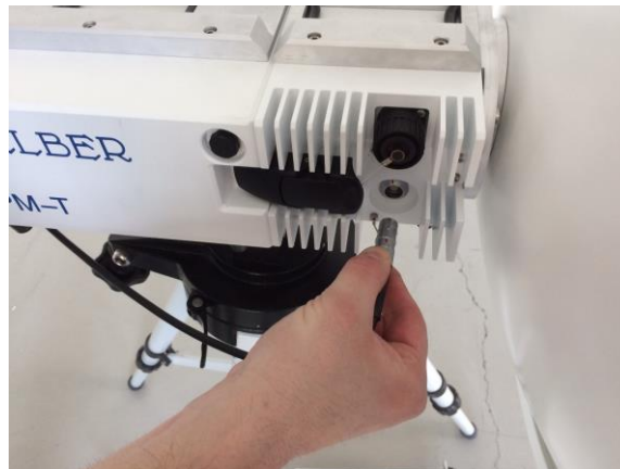
FIGURE 30: BOOSTER POWER SUPPLY CABLE CONNECTION B
